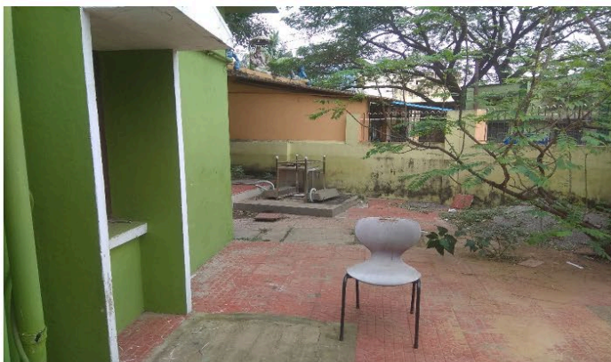
Handwash (Totally neglected condition)
